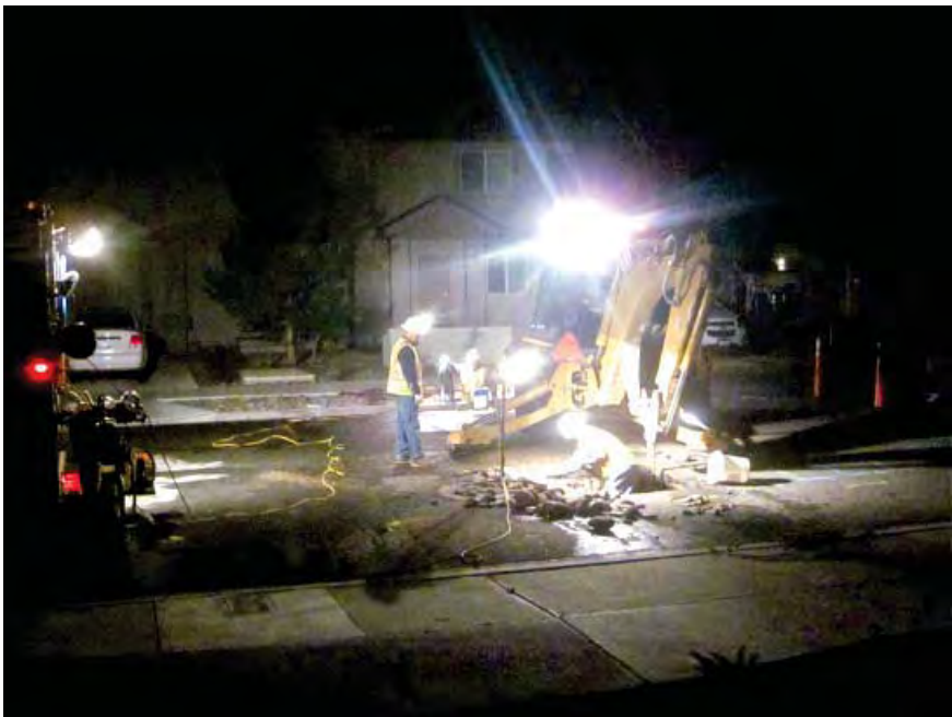
In the a.m. hours in downtown Sparks on April 17, residents were woken by a terrific racket. Truckee Meadows Water Authority workers were repairing an underground leak on 11th Street. By the time most people got up and were ready for showers, it was repaired. PHOTO/DENNIS MYERS
