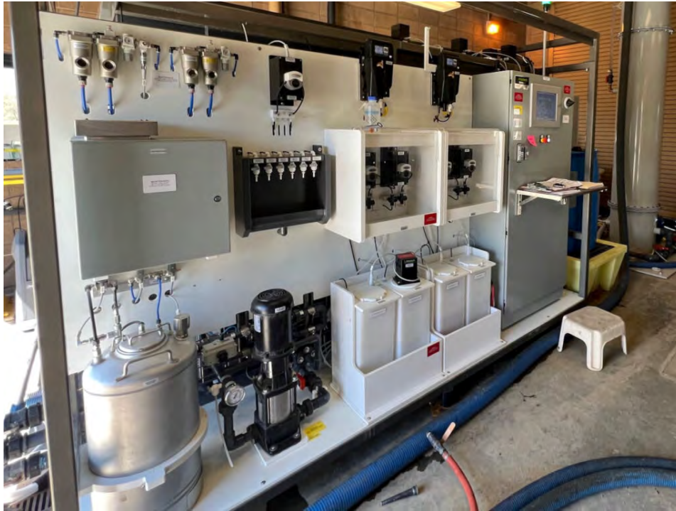
Dissolved air flotation equipment used by OneWater Nevada on a pilot study to test and evaluate water treatment design. Credit: OneWater Nevada.
