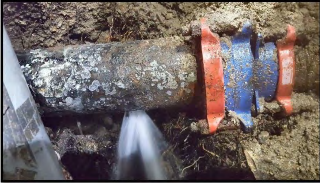
An example of an aging, burst pipe in the Rocky Point neighborhood. Provided/STPUD
