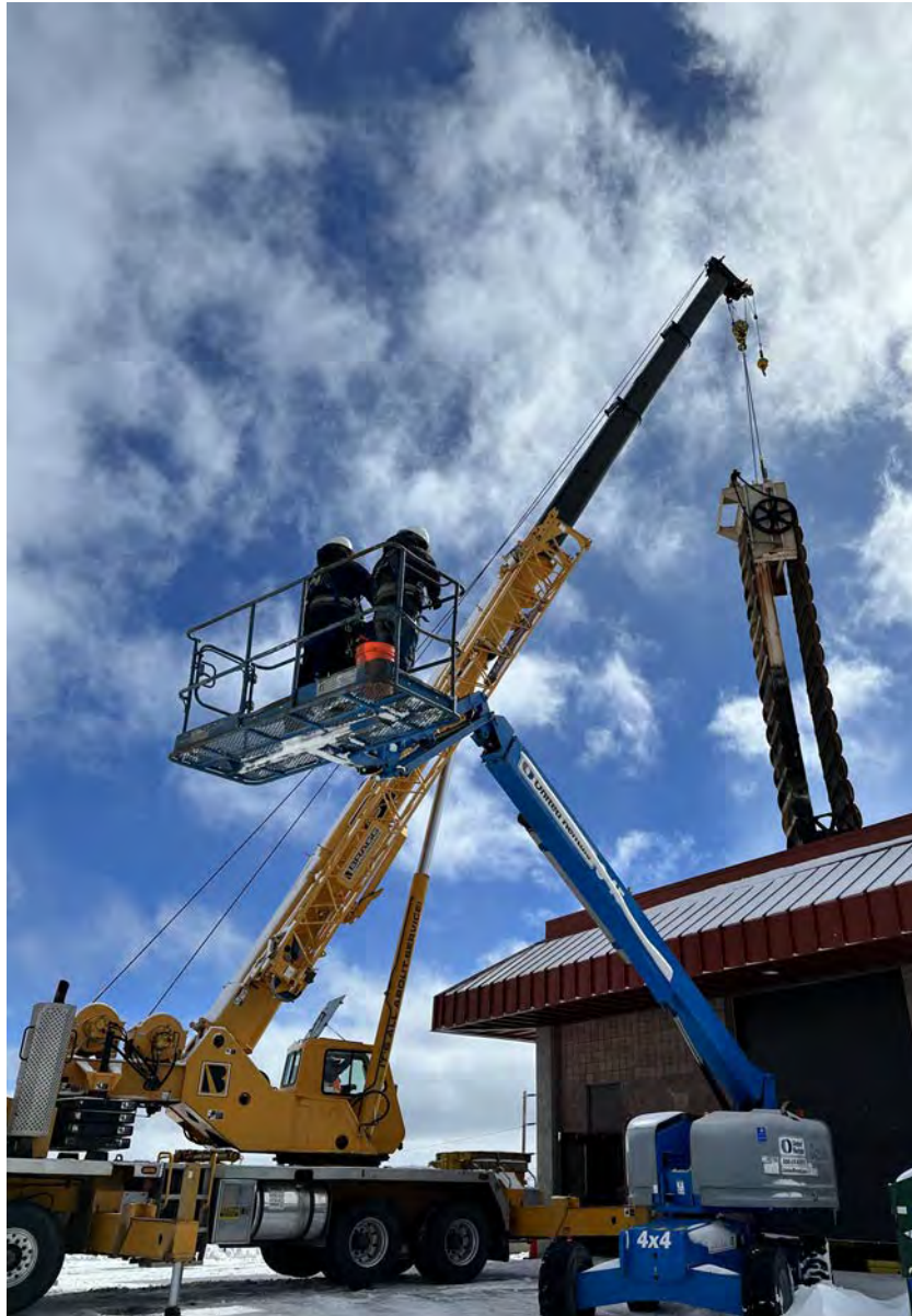
Photo: Traveling Screen 1 Rebuild, Chalk Bluff Water Treatment Plant Photo By: Jackie Heidelberger, Maintenance Supervisor
