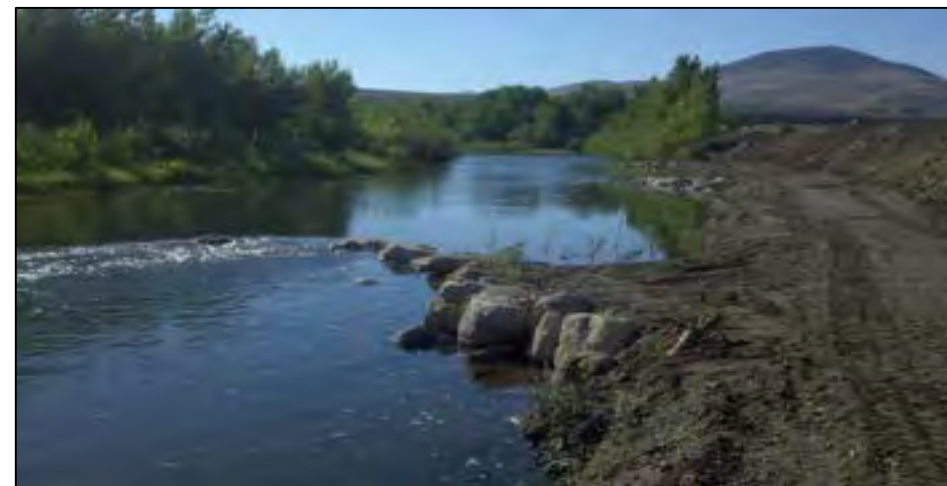
J-Hook Vane series following construction and willow planting Truckee River near Pyramid Lake
