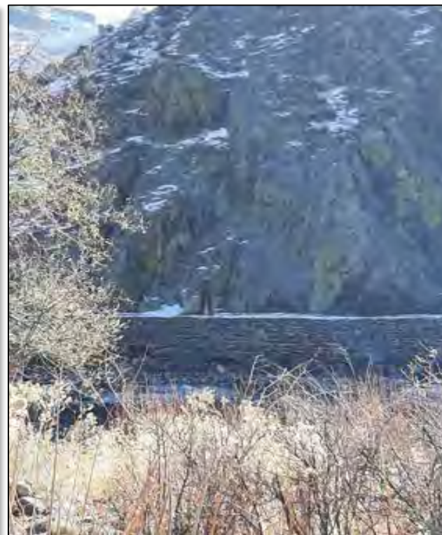
Historic rock wall undermined by flow.
