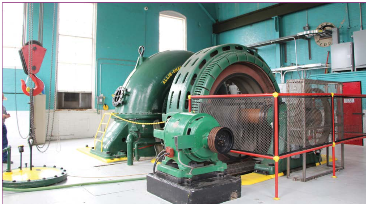
TURBINES AT VERDI HYDROELECTRIC PLANT
