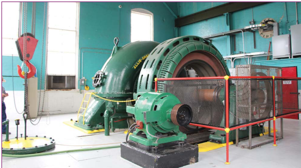
TURBINES AT VERDI HYDROELECTRIC PLANT
