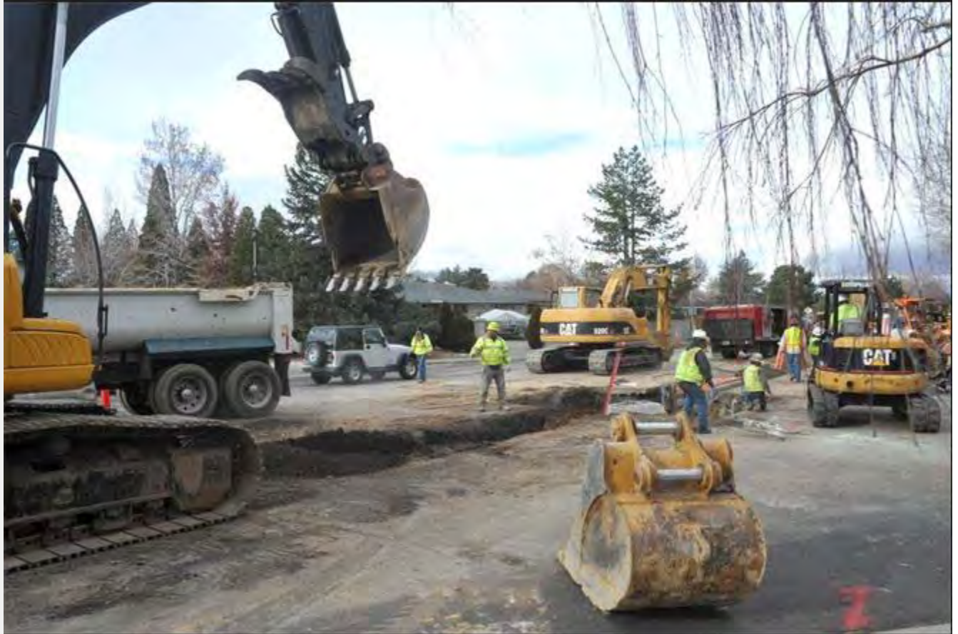
Crews install more sewer line capability on Plumas Street in 2010. (RGJ file)
