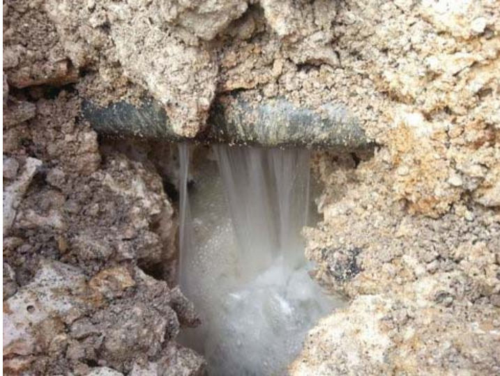
A cracked PVC pipe in an area of extremely high leakage in New Providence. Miya
