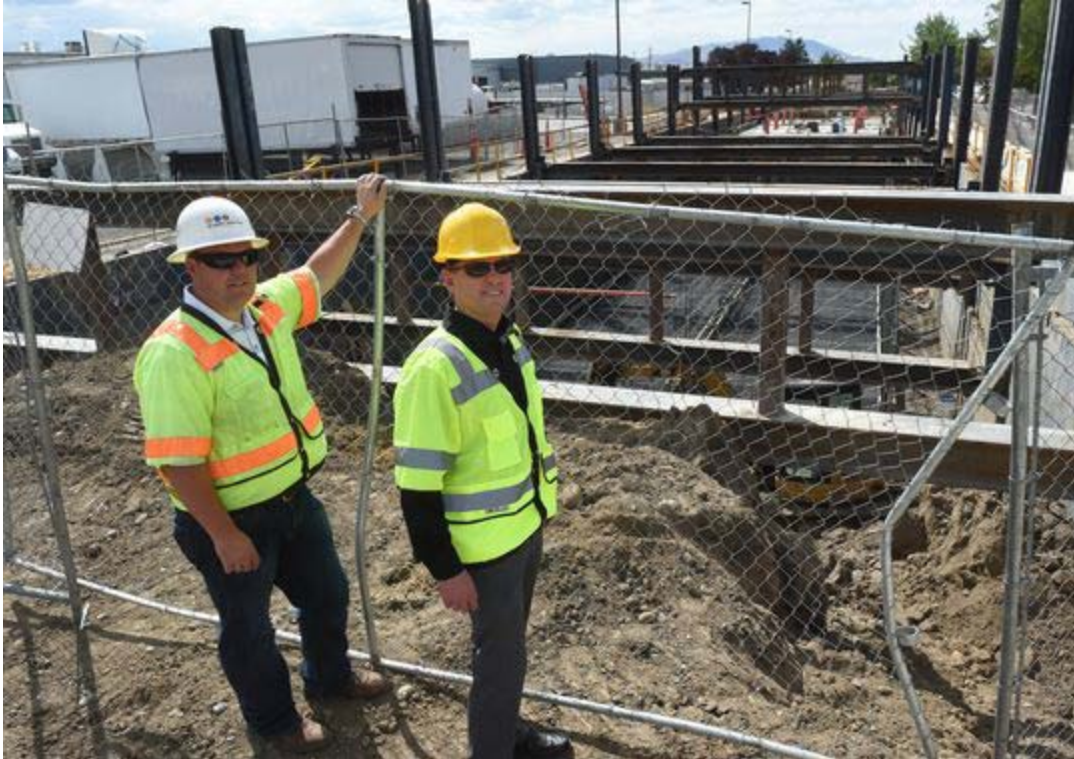
Andy Hummel, left, utility manager for the city of Sparks, and Sparks senior planner Jim Rundle pose in late July at the construction site for the North Truckee Drain culvert east of Greg Street. (Photo: Tim Dunn/RGJ)
