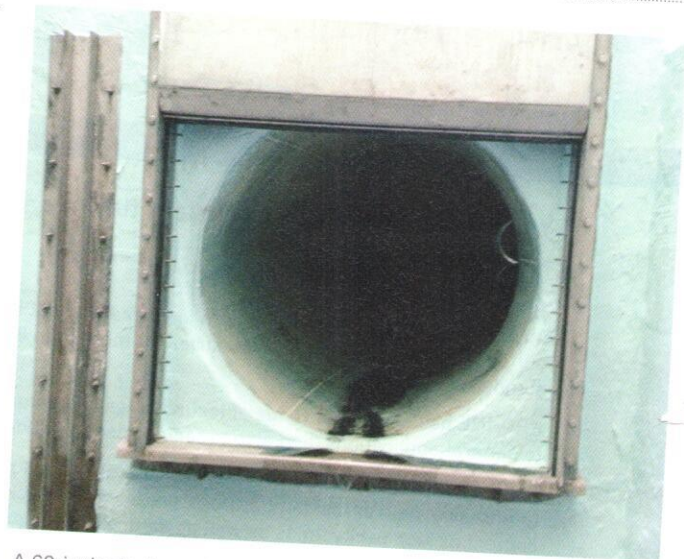
A 60-inch pipeline, with coated inlet structure, entering the Reno water treatment plant.
