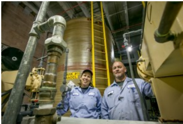
Sheryl Houlihan and Mike Witt in front of the 8,000-gallon “bleach tanks” that store the sodium hypochlorite used to disinfect the water.
