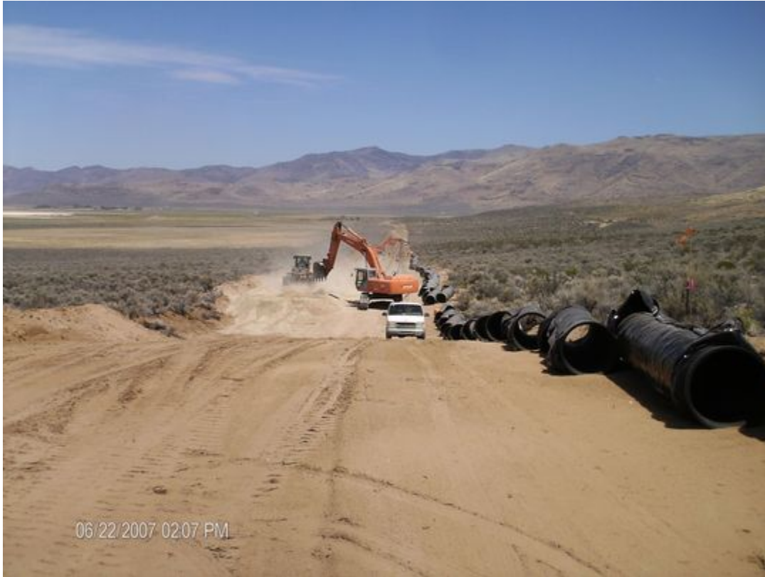
Excavation work is done in Dry Valley in June 2007 as part of the North Valleys Importation Project. (Photo: Provided by TMWA)
