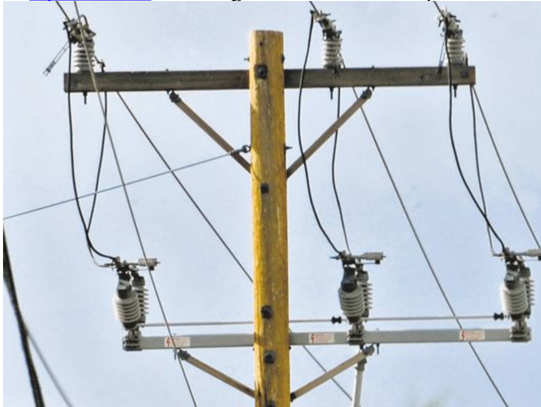
NV Energy power lines(Photo: RGJ file)
