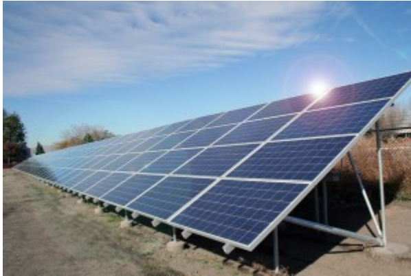
Solar Array located at TMWA’s Corporate Office
