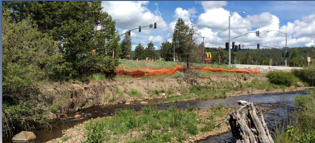
Eroding bank adjacent to Highway 89. Photo by Jai Singh, cbec (2015).
