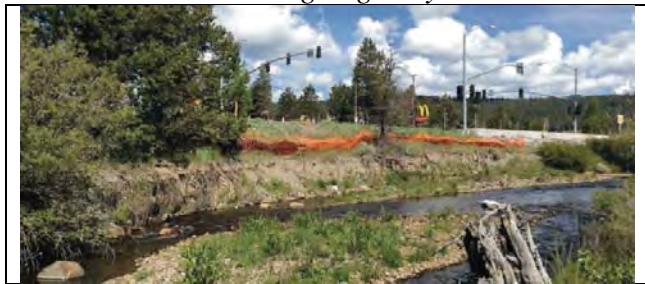
Project Site 1: Eroding bank along Highway 89
