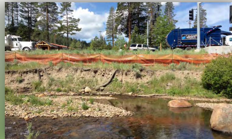
Eroding bank adjacent to Highway 89. Photo by Jai Singh, cbec (2015).
