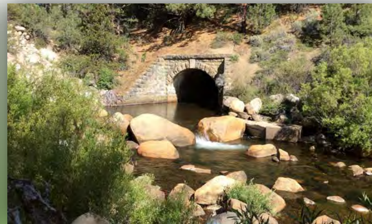
Railroad culvert just upstream of eroding bank. Photo by Jai Singh, cbec (2015).
