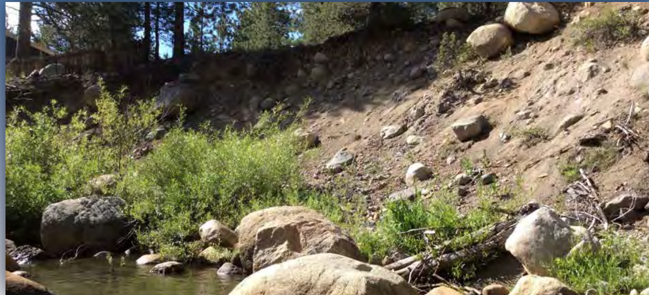
View of the upstream portion of the eroding bank. Photo by Jai Singh, cbec (2015).
