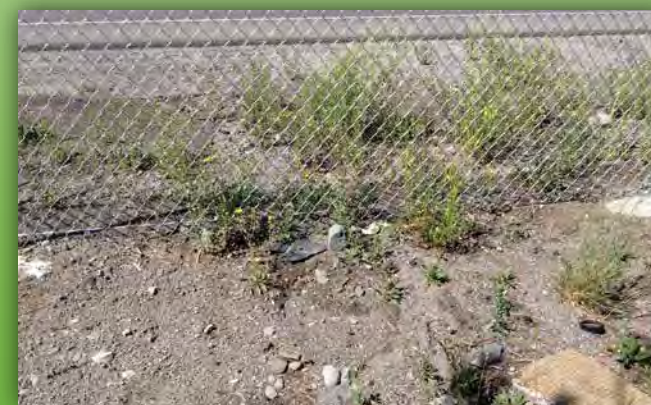
Localized erosion and debris from I-80 runoff. Photo by Jai Singh, cbec (2015).
