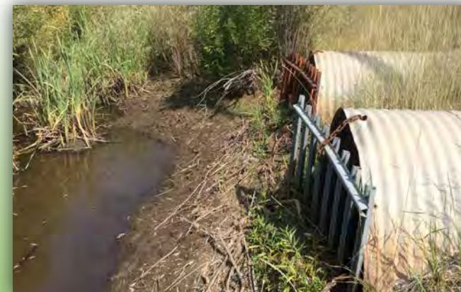
Sediment accumulation at culvert inlets which convey water to Donner Creek. Photo by Jai Singh, cbec (2015).
