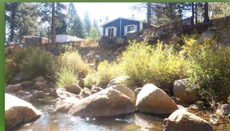
View of the downstream portion of the eroding bank. Photo by Jai Singh, cbec (2015).
